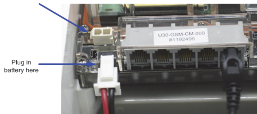
Connecting the Battery
