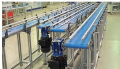
Figure 2.3 Monitoring vibration and temperature in conveyors.
