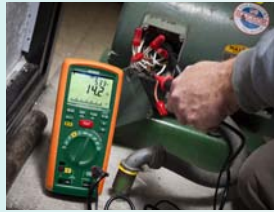
Insulation test on pump motor
