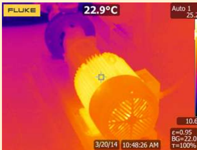
Combo: This heat pattern indicates an operational motor.
